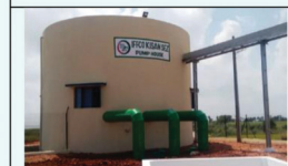
Pump House at Kanigiri Reservoir
